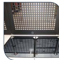
Data cage extends under flooring
