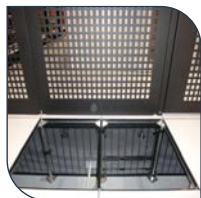
Data cage extends under flooring
