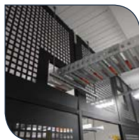
Cables into and out of data cage
