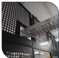
Cables into and out of data cage
