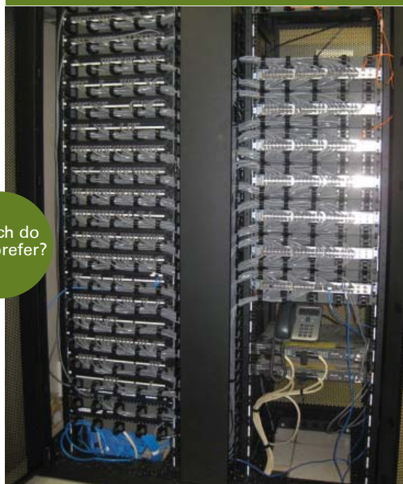
After using Ausrack Plus cable management system
