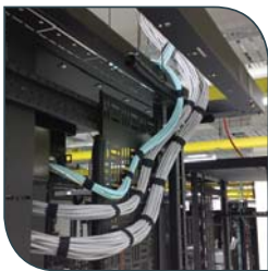
Side access for cable zones
