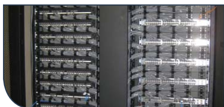
After cable management
