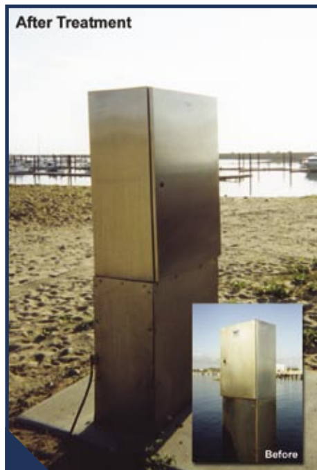
Figure 6 - Showing tea staining after treatment
